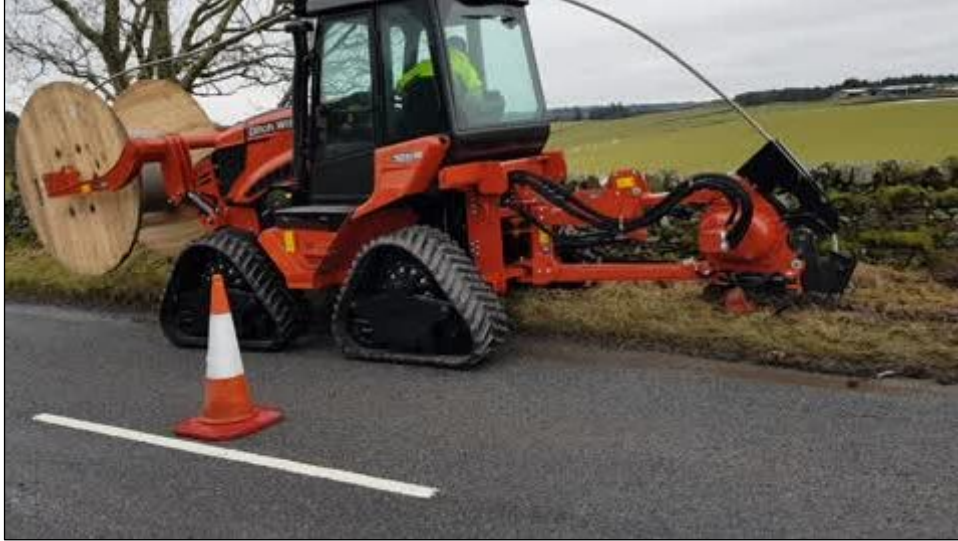
Photograph 2. Example of a running line installation using the plowing in method on the highway shoulder. Photograph taken on a different Zayo fiber optic project.
