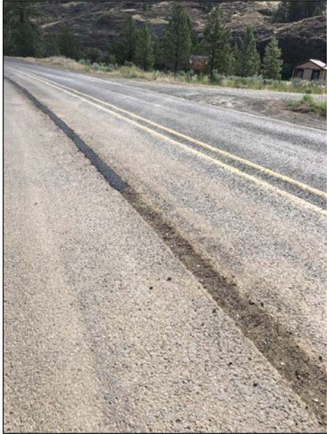
Photograph 1. Example of the running line installed into existing pavement. Photograph taken in a newly constructed portion of the project.
